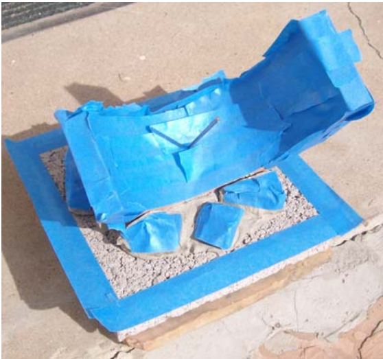
The dial protected with masking tape before mortar was applied. Mortar was used rather than sanded grout, this was to generate a coarser finish.
